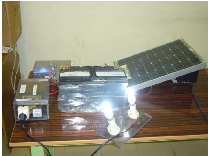
Figure 13. Complete intelligent system operation—Battery charge.
