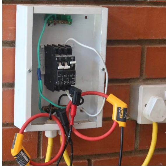
Figure 3. Single-phase connection of the power logger on the biodiesel processor breaker box.
