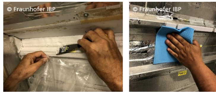
Figure 10. Collection of accumulated frost from the structure.
