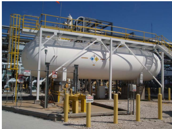
Figure 2. Cylindrical pressure vessel in a chemical plant.
