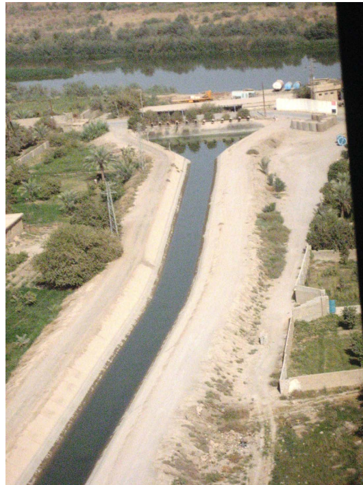
Figure 29. The Yusufiyah Tigris River feeder canal. A view from Pump Station #2. Photo credit: David R. Speidel, U.S. Department of Agriculture.
