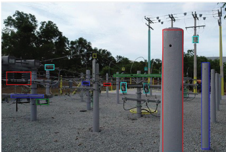
Figure 2. Electric network distribution components.
