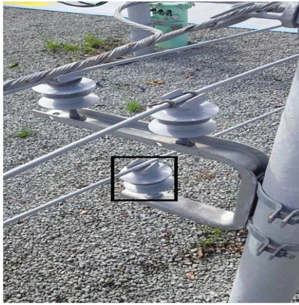
Figure 16. Isolator with no ring.
