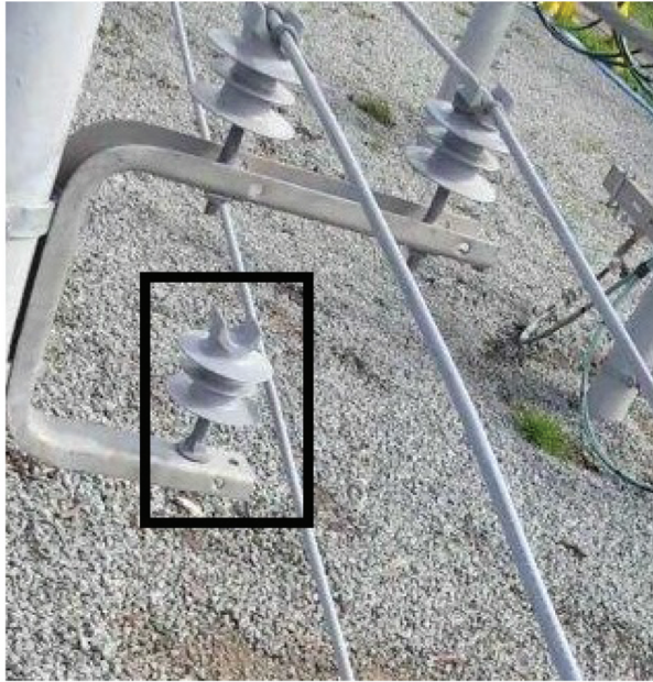
Figure 14. Cable out of isolator.
