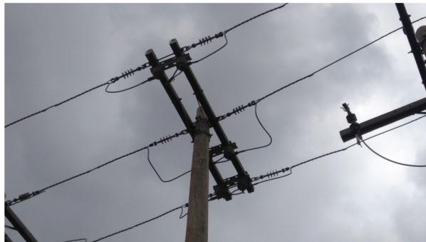
Figure 5. Section divider structure knife switch.
