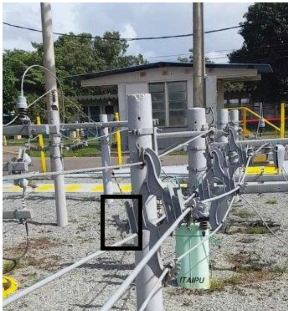
Figure 15. Cable out of spacer.
