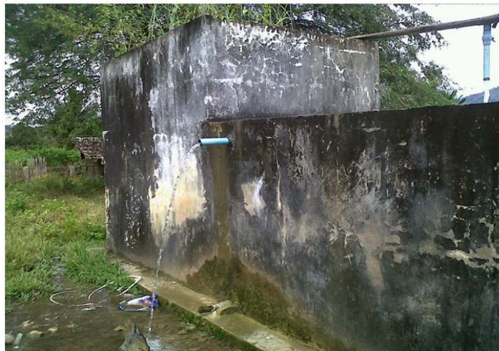
Fig. 3. Concrete water storage tank for the community and Buddhist monastery
